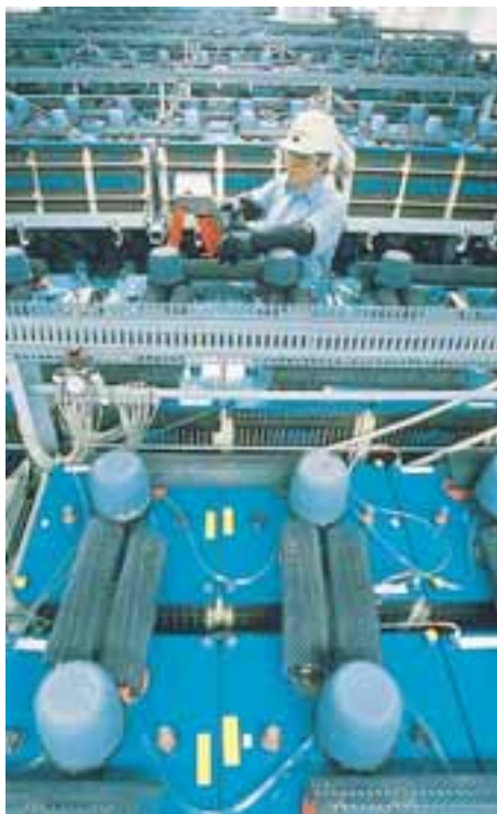
The world's largest battery energy storage plant (dismantled in 1996) connected over 8000 large lead-acid batteries in 8 strings at 1000 V each with a capability of 10 MW of power for 4 hours. Charged up at night, the batteries were then put to use during peak power demands on the electrical system. (Courtesy Southern California Edison Company)
