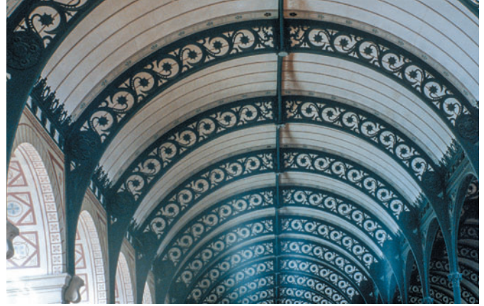
Figure 12.58 Sainte-Geneviève Library, Paris, France, Henri Labrouste, 1850. Decorative curved iron beams over the reading room.
