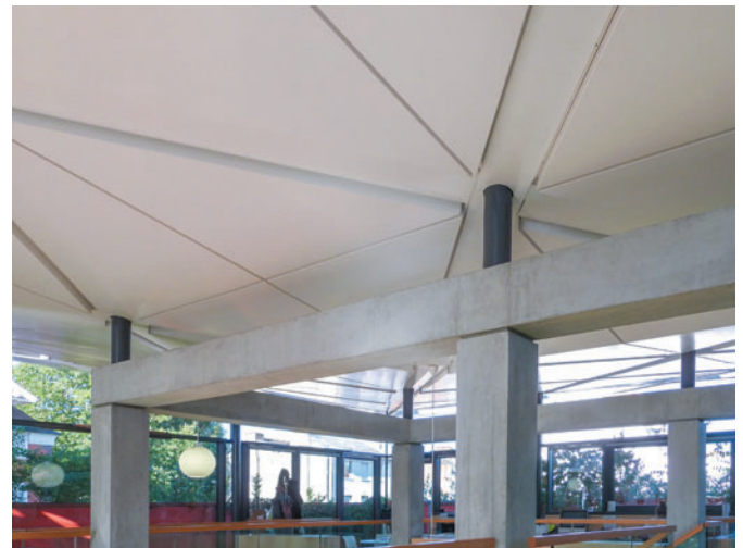
Figure 11.54 The roof is supported by fine steel tubes that raise it above the beams defining the core of the building.
