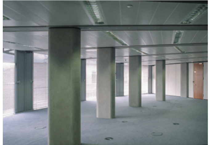
Figure 12.54 Generously chamfered interior columns reflect the curved plan shape of the new insertion. Partition walls are yet to be constructed.
