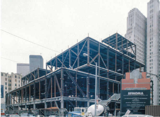
Figure 10.8 San Francisco Museum of Modern Art, San Francisco, USA, Mario Botta, 1995. The structural steel framework during construction.
