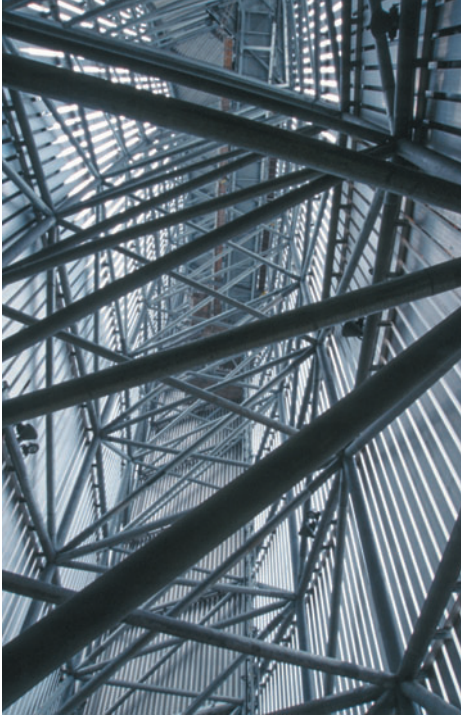
Figure 9.28 Imperial War Museum-North, Manchester, UK, Studio Daniel Libeskind, 2002. Structural members dominate the Air Shard volume.
