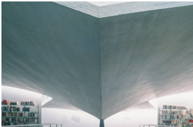
Figure 12.32 Wöhlen High School, Switzerland, Santiago Calatrava, 1988. Concrete roof structure over the library.
