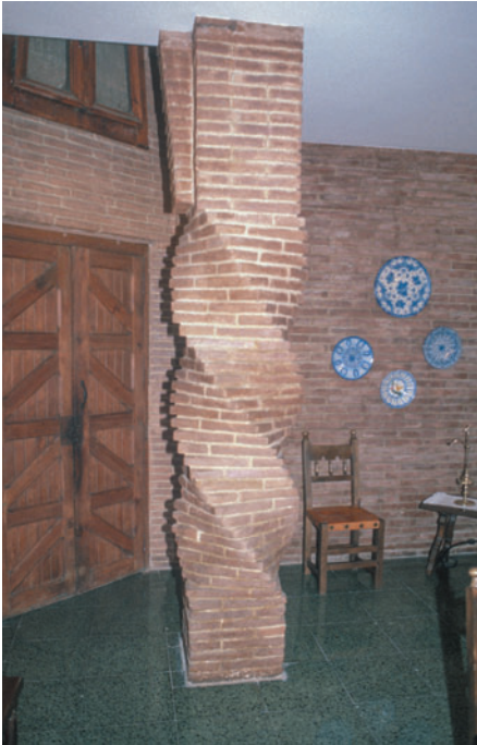
Figure 10.14 Colegio Teresiano, Barcelona, Spain, Antoni Gaudí, 1889. A spiral brick masonry column that is not immediately recognized as structure.
