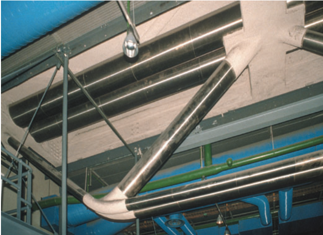
Figure 12.26 Centre Pompidou, Paris, France, Piano and Rogers, 1977. Double-chords reduce the visual mass of the truss.
