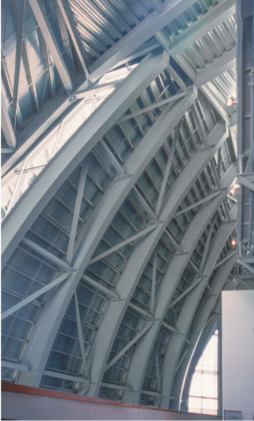
Figure 7.30 Exposed construction of an exterior wall that curves towards the theatre roof.
