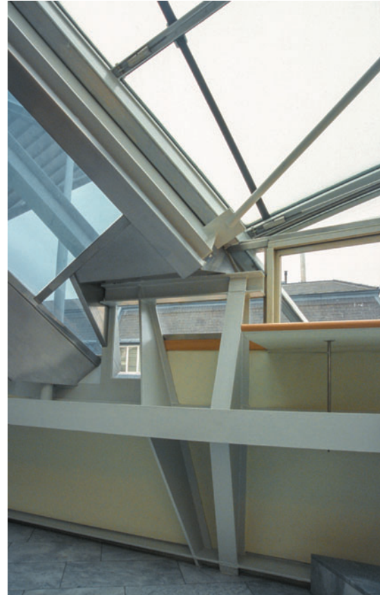
Figure 12.61 Irregularity of the form is reflected in the roughness of the detailing.
