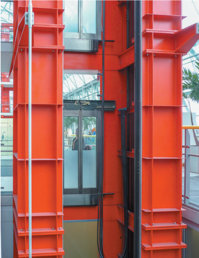
Figure 7.19 Towers express steel construction through the use of steel plates and stiffeners.
