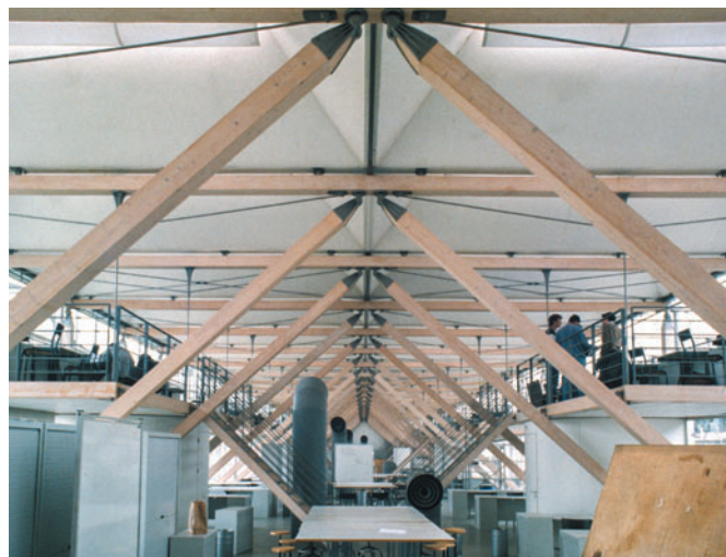
Figure 6.19 Lyon School of Architecture, Lyon, France, Jourda et Perraudin, 1988. Structure breaks up a large studio area.
