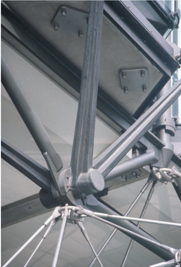
Figure 12.53 Bracken House, London, UK, Michael Hopkins and Partners, 1991. Elegant truss members meet at a joint.
