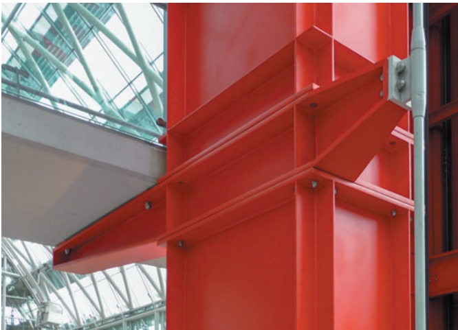
Figure 7.20 Bolts clamp tower sections together and a double-cantilevered beam supports a concrete bridge slab at one end and is held down at the other by a tensioned rod anchored in the foundations.
