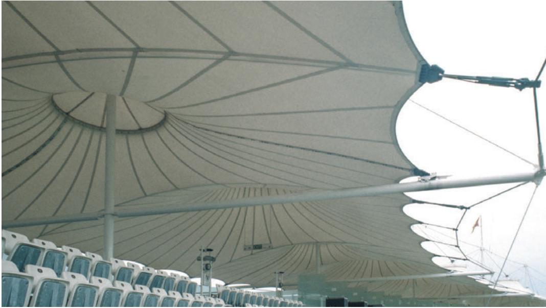
Figure 8.36 Mound Stand, Lord's, London, Michael Hopkins and Partners, 1987. Underside of the fabric roof.
