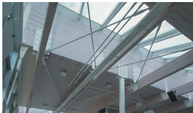
Figure 8.34 Business School, Öhringen, Germany, Günter Behnisch & Partner, 1993. A primary beam with the skylight above and the roof below.
