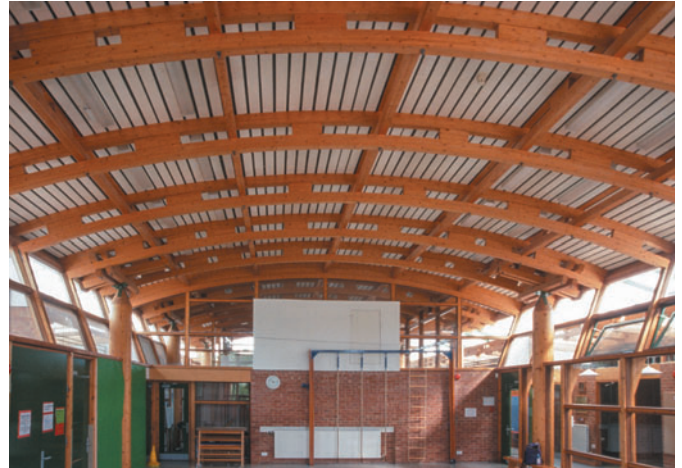
Figure 7.21 Hazel Wood School, Southampton, UK, Hampshire County Council Architects Department, 1990. The hall roof structure is typical of that for the whole school.
