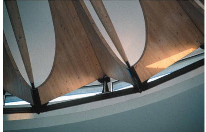
Figure 6.2 Refined wooden struts connect to the steel rod tension-ring and the rafters with deepened ends.
