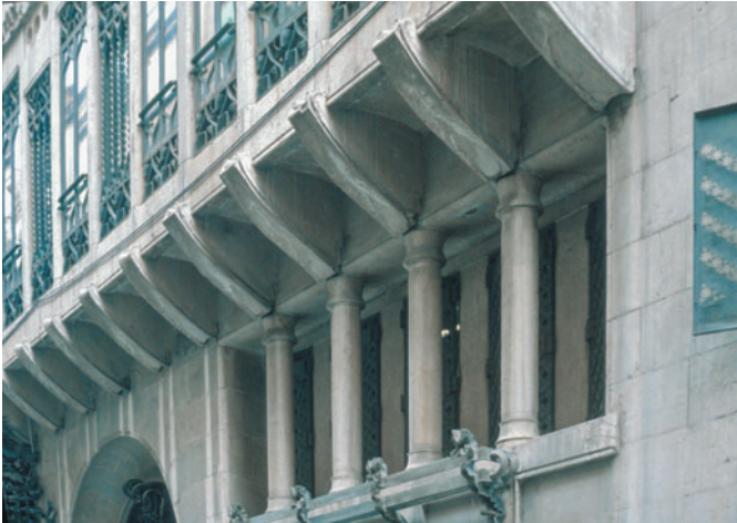
Figure 7.40 Palau Güell, Barcelona, Spain, Antoni Gaudí, 1880. Cantilevering brackets clasp the oriel floor.
