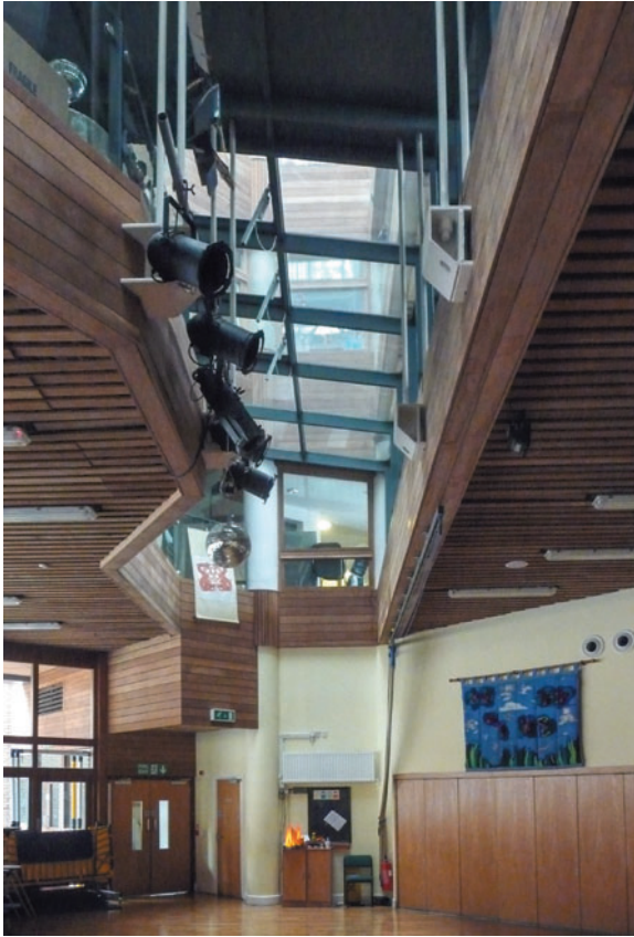
Figure 5.3 Hampden Gurney Church of England Primary School, London, UK, Building Design Partnership, 2002. The assembly hall. Four pairs of hanger rods transfer forces from the floors above up to the roof-top transfer structure.
