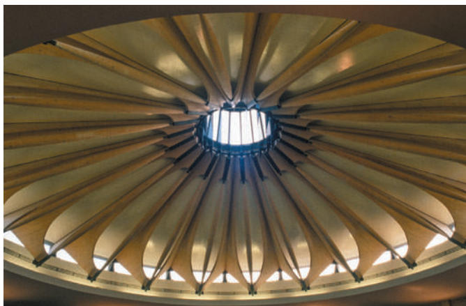
Figure 6.1 Wöhlen High School, Switzerland, Santiago Calatrava, 1988. Attractive structural framing pattern of the entrance foyer roof.
