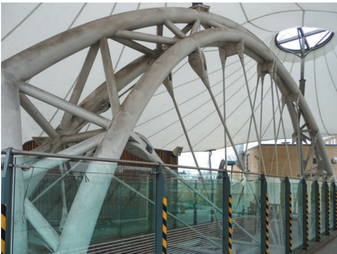
Figure 5.4 Inclined tension rods connect into the arched truss which also supports the two high points of a tension-membrane roof canopy.
