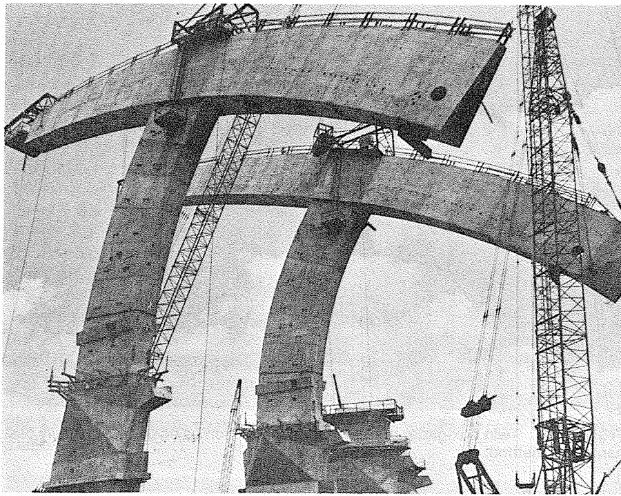
FIGURE 1.6 Segmentally precast post-tensioned rigid frames for the Olympic stadium in Montreal. Photograph courtesy of Regis Trudeau and Associates, Inc., Montreal, Canada.
