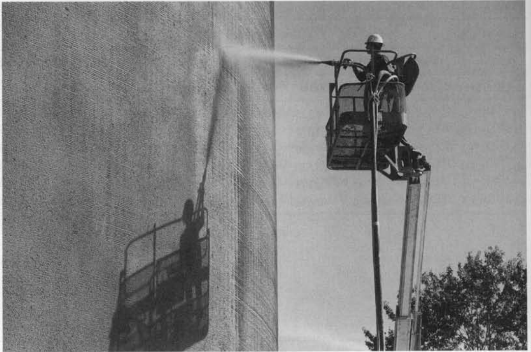
Photo 11.7 Shotcrete Application Covering the Wire (Courtesy, N.A. Legatos, Preload Inc., Garden City, New York.)
