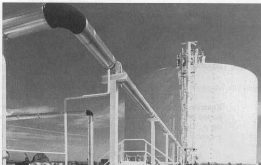
Photo 11.3 250,000-bbl (39,750-m 3 ) prestressed concrete propane gas storage container, Winnipeg, Manitoba, Canada. (Courtesy, N.A. Legatos, Preload Technology, Inc., New York.)
