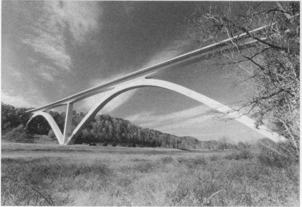
Photo 12.7 Natchez Parkway Arches, Nashville Tennessee, America's first segmental arch bridge; principal arch span is 582-ft. long and has a vertical clearance of 137 ft (Courtesy Figg Engineering Group, Tallahassee, Florida)
