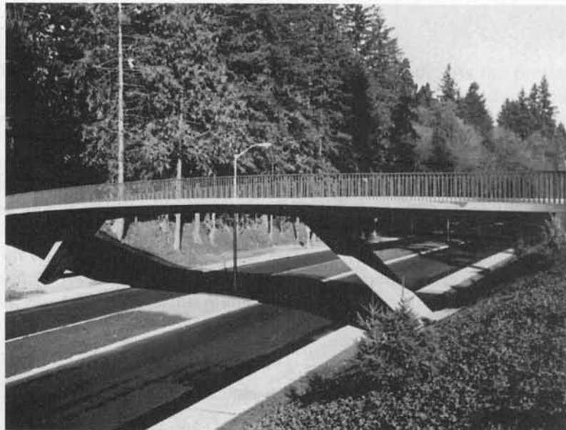
Photo 7.2 Priest Point Park Bridge in Olympia, Washington, a cast-in-place prestressed concrete structure. (Courtesy, Arvid Grant and Associates, Inc.)
