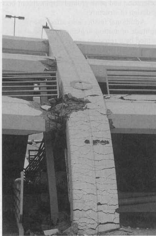
Photo 13.3 Northridge, California, 1994 earthquake structural failure. (Courtesy Dr. Murat Saatcioglu.)
