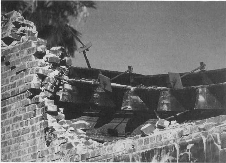
Photo 13.9 Masonry collapse in Los Angeles earthquake, 1994. (Courtesy Portland Cement Association.)
