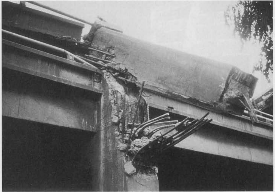
Photo 13.2 Bridge girder collapse in the San Francisco 1989 earthquake. (Courtesy Portland Cement Association.)
