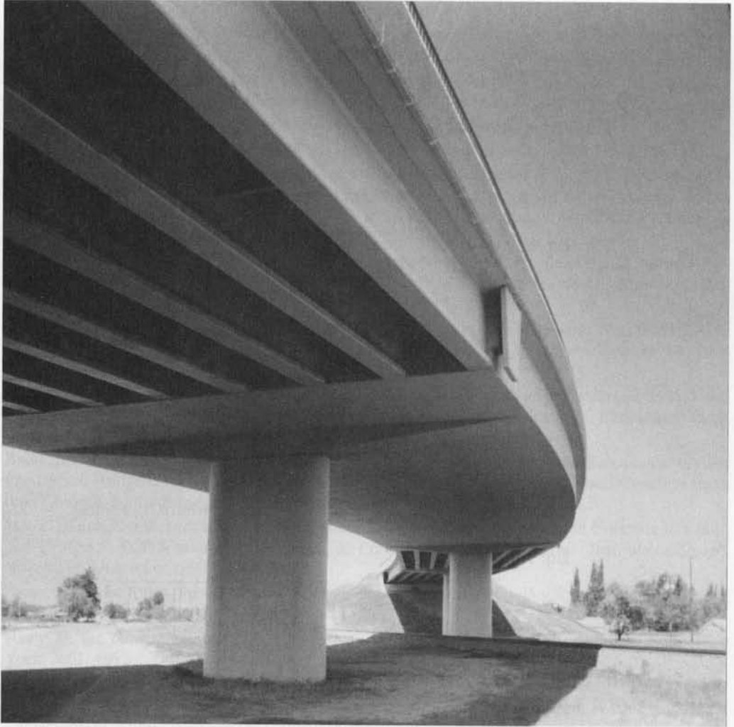
Photo 12.11 Valley Ave. Bridge, Fife, Washington: 4-span bridge consisting of two structural types, situ-cast post-tensioned concrete box girder with precast prestressed end girders (Designed by BERGER/ABAM Engineers, Federal Way, Washington, courtesy Robert Mast, Senior Principal)
