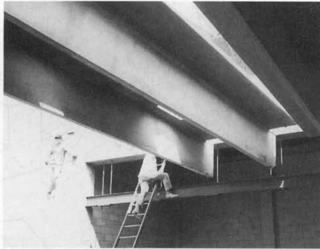
Photo 10.7 Installation of prestressed double-T elements at the rod-suspended support, Civil Engineering Laboratory, Rutgers University.
