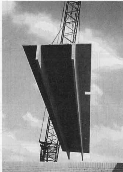
Photo 10.5 Hoisting double-T prestressed roof element at the Civil Engineering Laboratory, Rutgers University.
