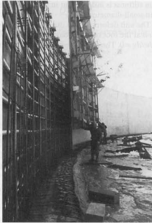
Photo 11.8 Six-million-gallon tendon-prestressed circular tank seen from inside with situ-cast walls. (Courtesy, Jorgensen, Hendrickson and Close, Inc., Denver, Colorado.)
