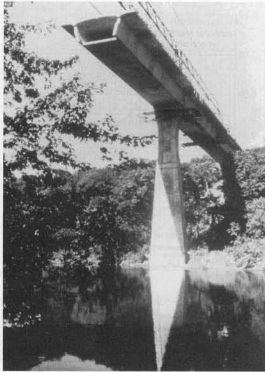
Photo 9.2 Kishwaukee River segmental bridge during construction. Winnebago County, Illinois. The first bridge in the U.S. constructed with launching gantry and the only precast segmental bridge post-tensioned totally with Dywidag bars. (Courtesy, H. Wilden & Associates, Macungie, Pennsylvania and the Prestressed Concrete Institute.)
