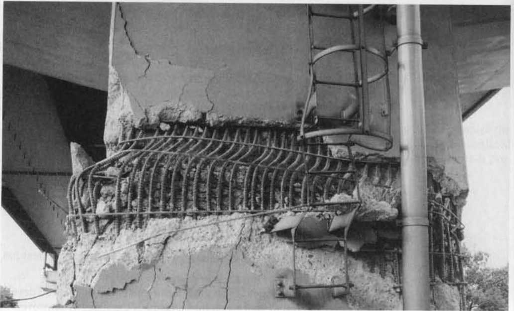
Photo 13.14 Failure of piers at Hanshin Highway Bridge, Kobe Earthquake, Japan, 1995 (Courtesy Professor Megumi Tominaga, Kyoto University, Japan)
