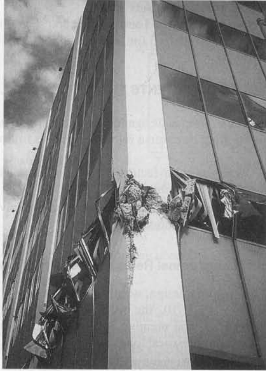
Photo 13.5 Column localized damage in a high-rise frame building, Los Angeles 1994 Earthquake. (Courtesy Portland Cement Association.)
