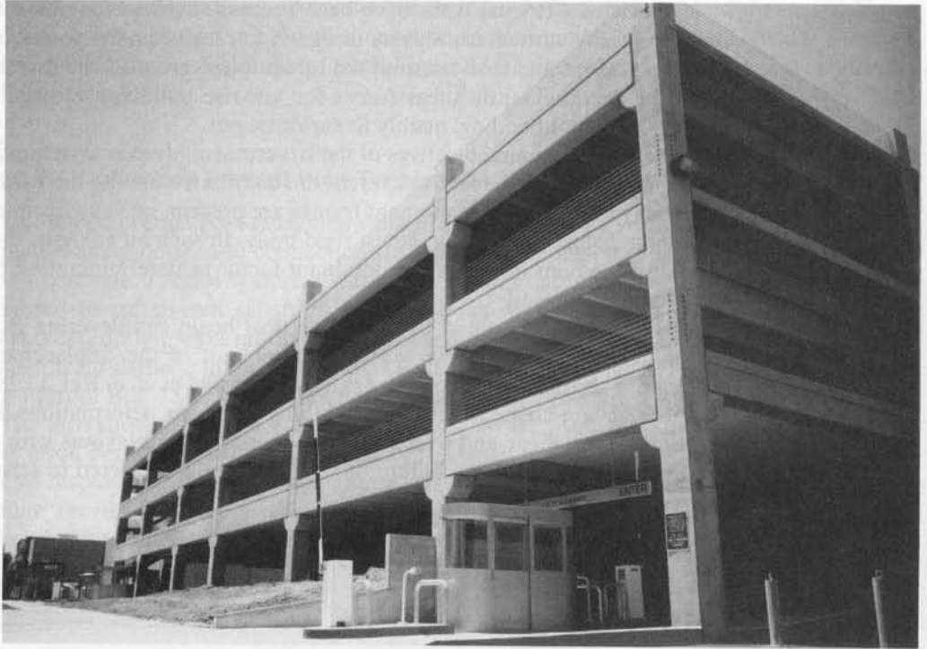
Photo 13.7 Wilern Center Parking Structure, Los Angeles, California (Courtesy Dr. Robert E. Englekirk).
