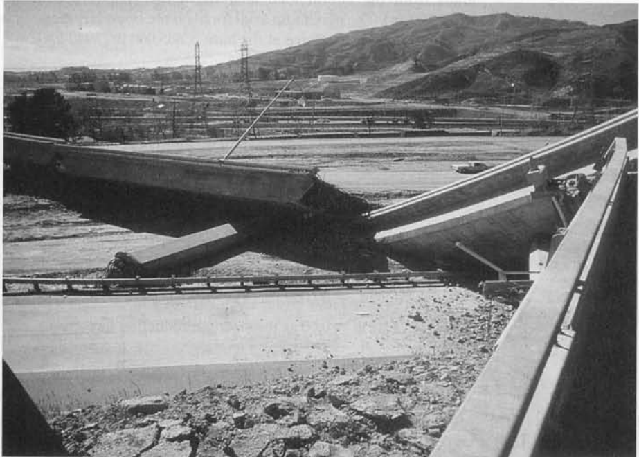
Photo 13.10 Overpass collapse in 1971 Los Angeles earthquake. (Courtesy Portland Cement Association.)
