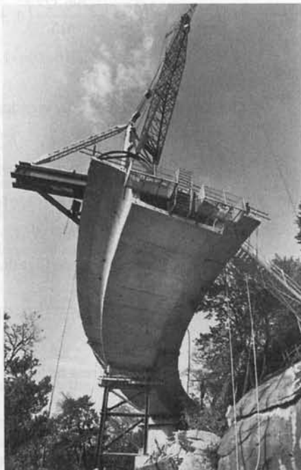
Photo 3.3 Linn Cove Viaduct, Grandfather Mountain, North Carolina. A 90° cantilever and a 10 percent superelevation in one direction to a full 10 percent in the opposite direction within 180 ft. Designed by Figg and Muller Engineers, Inc., Tallahassee, Florida. (Courtesy, Figg and Muller Engineers, Inc., now FIGG Engineers)
