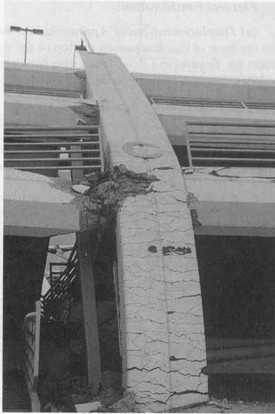
Photo 13.6 Northridge, California, 1994 earthquake structural failure. (Courtesy Dr. Murat Saatcioglu.)
