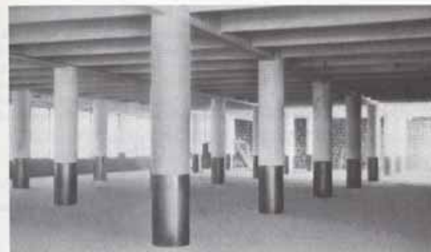
Monolithic slab—beam—girder system; Liggett and Myers Tobacco Company, Richmond, VA. (Courtesy of Portland Cement Association.)
