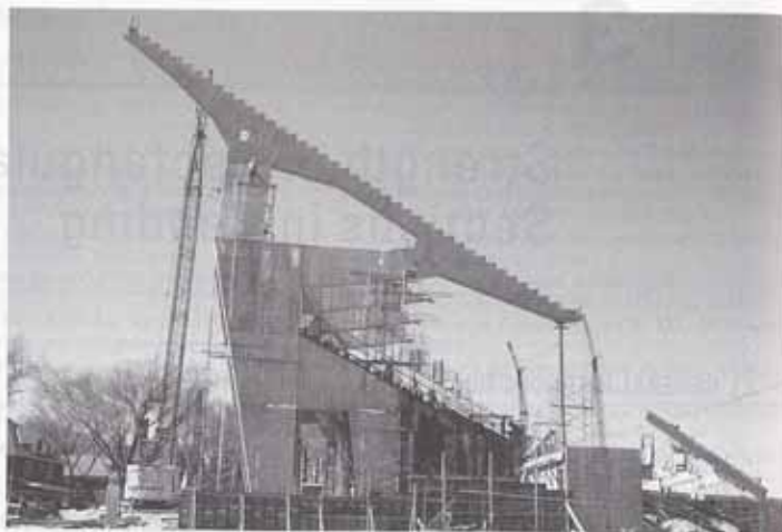
Rectangular tapered beams, cantilevers, and rigid frame. University of Wisconsin Stadium, Madison, WI. (Photo by C. G. Salmon.)
