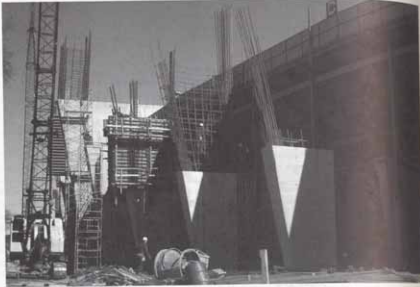
Construction of tapered rigid frame knee for University of Wisconsin Stadium. (Photo by C. G. Salmon.)
