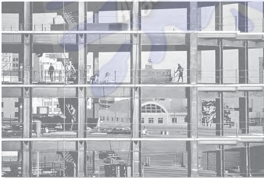
The building framework has rigid connections. A lateral-load analysis can be performed (approximately) by using the cantilever method of analysis.
