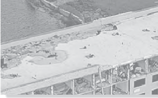
Hurricane winds caused this damage to a condominium in Miami, Florida.
