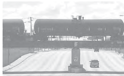
The absolute maximum moment in this girder bridge is the result of the moving concentrated loads caused by the wheels of these train cars. The cars must be in the critical position, and the location of the point in the girder where the absolute maximum moment occurs must be identified.
