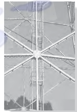
The gusset plate is used to connect eight members of the truss supporting structure for a water tank.
