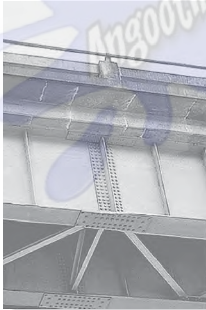
Shown are typical splice plate joints used to connect the steel girders of a highway bridge.
