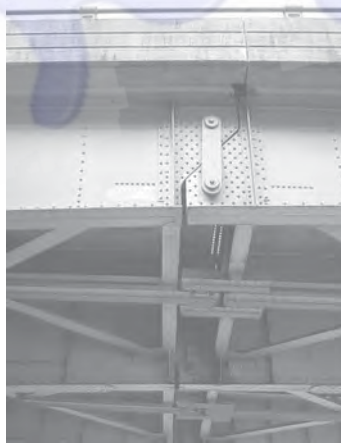
The short link is used to connect the two girders of the highway bridge and allow for thermal expansion of the deck.
