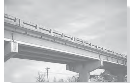
The prestressed concrete girders are simply supported and are used for this highway bridge.
