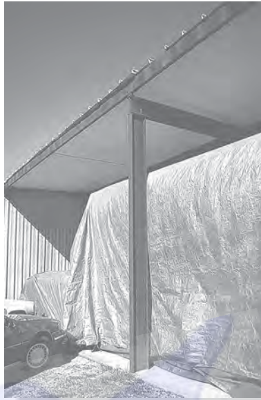
Wide-flange members are often used for columns. Here is an example of a beam column.
