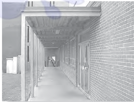
The two-member frames support both the dead load of the roof and a live snow loading. The frame can be considered pinned at the wall, fixed at the ground, and having a fixed-connected joint.
