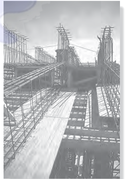
The steel reinforcement cage shown on the right and left is used to resist any tension that may develop in the concrete beams which will be formed around it.
