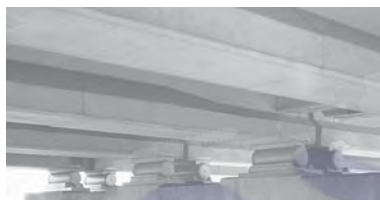
Rollers and associated bearing pads are used to support the prestressed concrete girders of a highway bridge.
