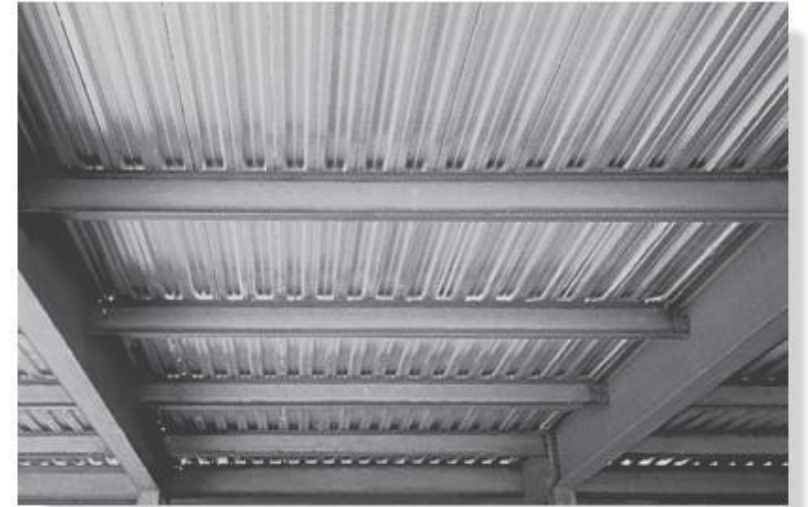
An example of one-way slab construction of a steel frame building having a poured concrete floor on a corrugated metal deck. The load on the floor is considered to be transmitted to the beams, not the girders.
