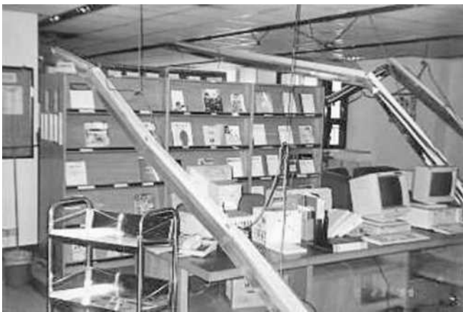
FIGURE C13.1-3 Collapsed Light Fixtures
