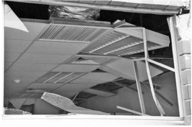
FIGURE C13.1-2 Damaged Ceiling System
