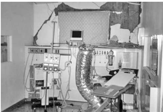
FIGURE C13.1-5 Collapsed Duct and HVAC Diffuser
