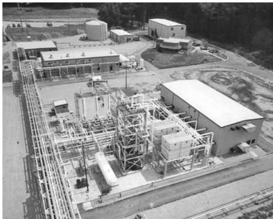
FIGURE C15.1-2 Steel pipe rack
