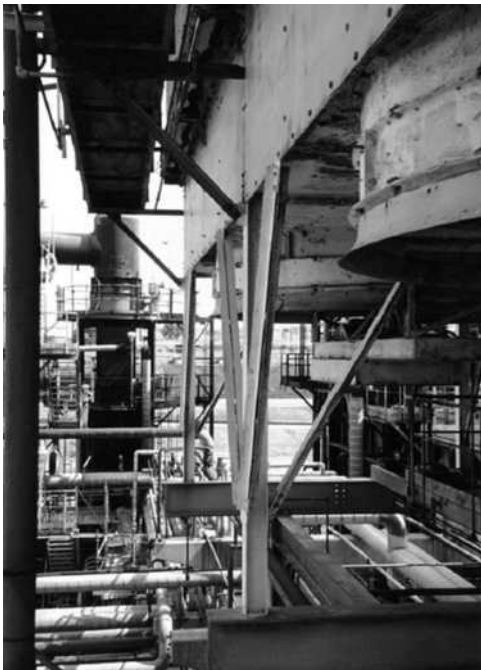
FIGURE C13.6-1 Fin Fan Elevated on Integral Supports
