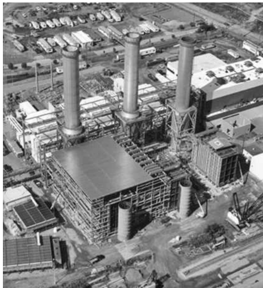
FIGURE C15.1-3 Heat recovery steam generators
