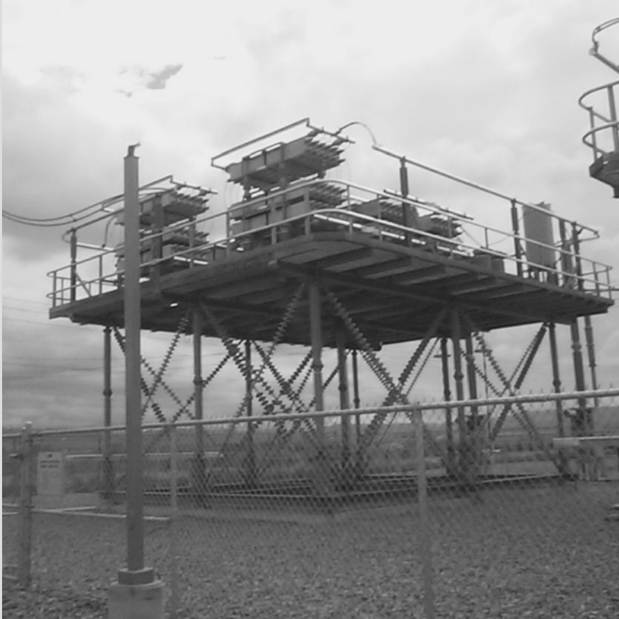
Series capacitor installation at Goshen Substation, Goshen, Idaho, USA rated at 395 kV, 965 Mvar (Courtesy of PacifiCorp.)
