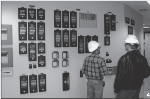
Figure 4 The old EM transformer differential relays (Photo courtesy of Basler Electric Company.)
