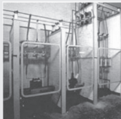
Figure 3 Air-insulated masonry cubicles
