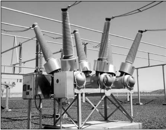
Figure 6 Dead tank circuit breaker 145 kV with spring-operating mechanism and double motion self blast interrupting chambers (Courtesy of Alstom Grid)
