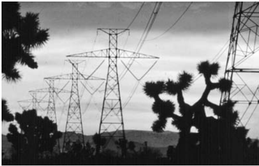
Figure 2 A ±500-kV HVDC transmission line
