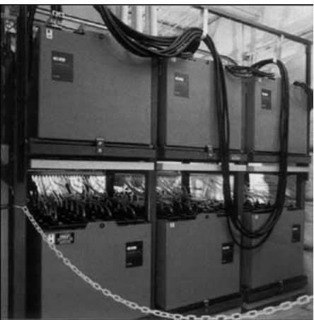
Figure 6 Large lead-acid battery bank
