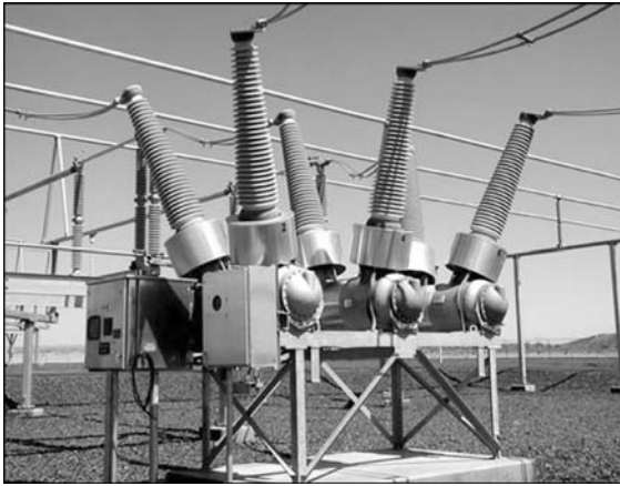
Figure 6 Dead tank circuit breaker 145 kV with spring-operating mechanism and double motion self blast interrupting chambers (Courtesy of Alstom Grid)
