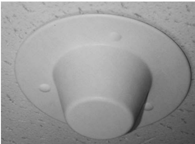
Figure 15.21: Typical ceiling-mounted indoor antenna (Reproduced by permission of Jaybeam Wireless)
