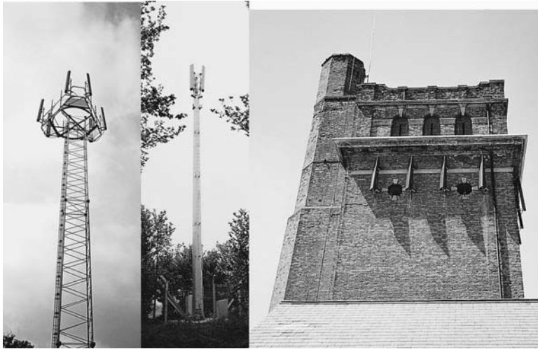
Figure 15.17: Typical macrocell installations (Reproduced by permission of O 2 (UK) Ltd.)
