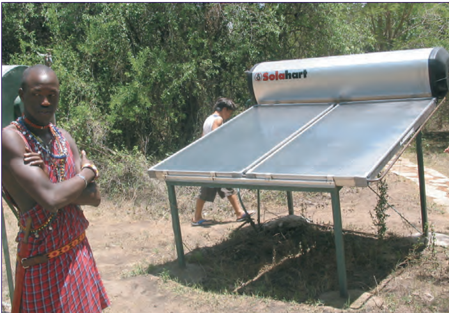
Figure 2.14 Solar water-heater in Maasai Mara, Kenya
