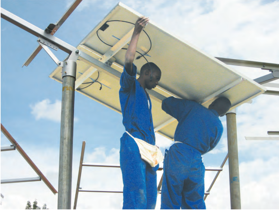
Figure 9.4 Working on roofs can be hazardous; the workers in this photo are taking unnecessary risks. Use a safety harness if there is a risk of falls, and protective headgear when manoeuvring large modules and mounting structures into place (see section on safe working practices, pages 144–146).
