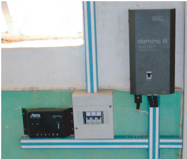
Figure 5.4 Charge controllers, MPPTs, main switches, inverters, fuse boards and other accessories on wall-mounted panels
