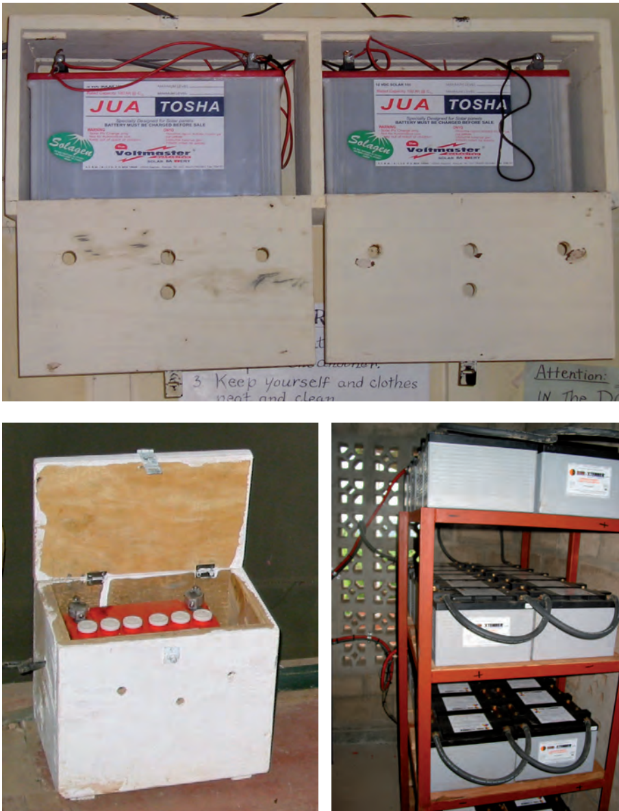
Figure 9.10 Battery box, rack and shed
