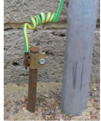
Figure 7.11 Earth rod connection
