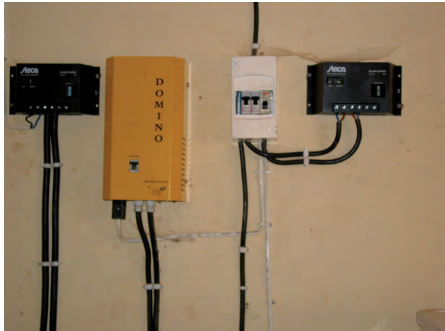
Figure 9.13 Charge controllers, main switch and monitor on sub-board
