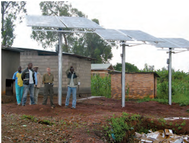
(b) Pole-mounted panels at a health centre in Rwanda (Walt Ratterman is second from right)
