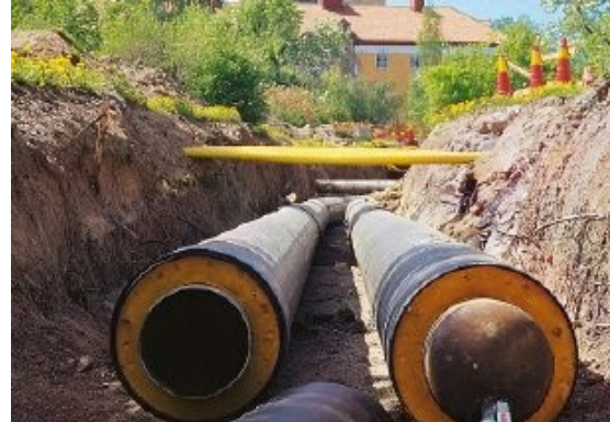
Pipes in the ground for distribution
