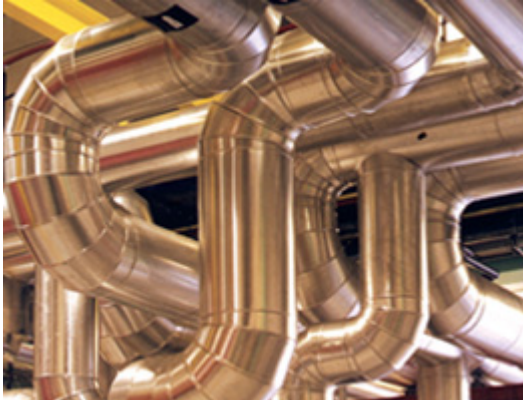
Pipes in the power plant
