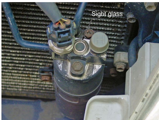
Figure 52-31 The location of a typical sight glass.
