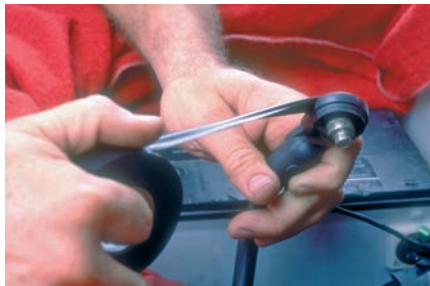
P22-5 Tape the cable terminal to prevent accidental connection with the battery post. Note: A piece of rubber hose can be substituted for the tape.
