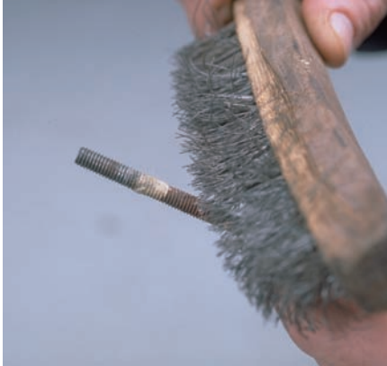
P5-10 Use a scraper and wire brush to remove corrosion from the hold-down hardware.
