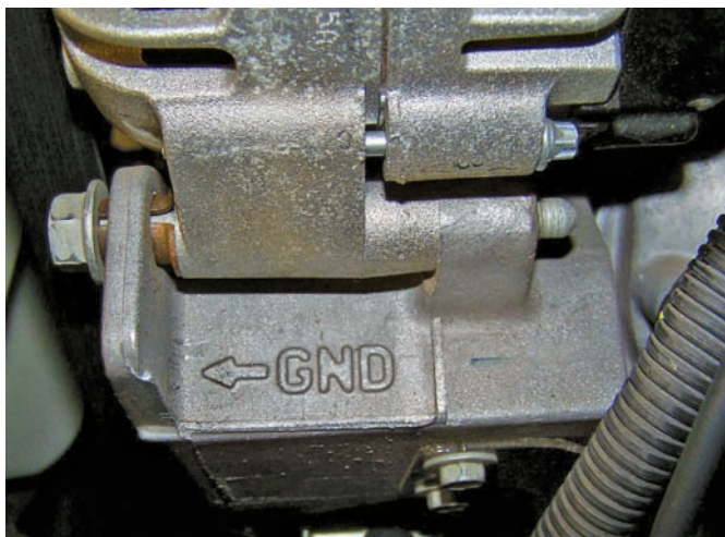
Figure 15-15 Many electrical parts are grounded through their mounting to the engine, transmission, or frame.
