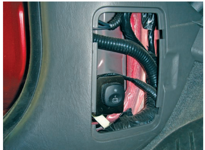
Figure 17-54 To jump-start a Ford Escape or Mariner hybrid high-voltage battery, turn the ignition off , open the access panel on the driver's side foot well, and press the jump-start button.
