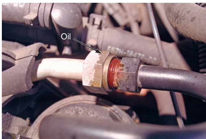
Figure 53-4 The oily film by this fitting is evidence of a refrigerant leak.
