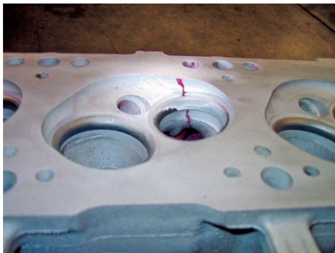
Figure 10-39 Cracks appear as red lines when a dye penetrant is used. Courtesy of LOCK-N-STITCH Inc.
