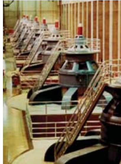
A series of hydel generators.
