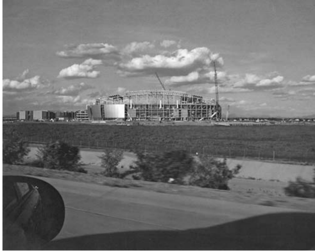
Figure 5–1 The Arizona Cardinal Football Stadium under construction—a rigid building frame (Courtesy Ed Yack)
