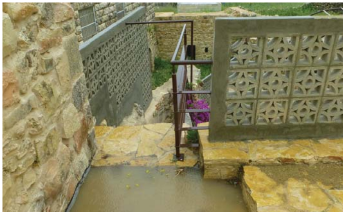
4. Periodic cleaning of gutters and drainpipes may prevent the risk of infiltration and stains on interior surfaces due to water stagnation.
