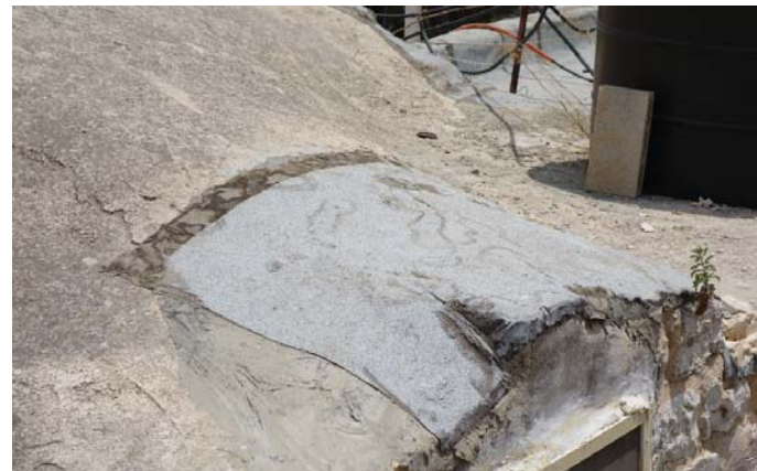
5. Periodic maintenance of the roof rendering may prevent infiltration through the roof structure, which can result in serious damage.
