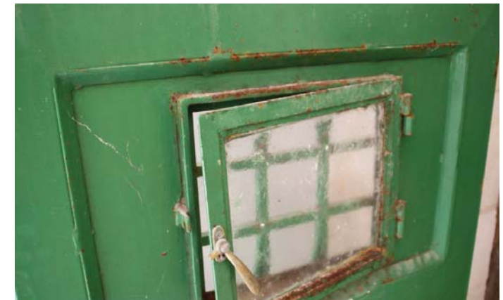
6. Quickly and duly fixing of any deteriorate building component is essential to preserve the building as a whole and ensure good life quality to the users.
