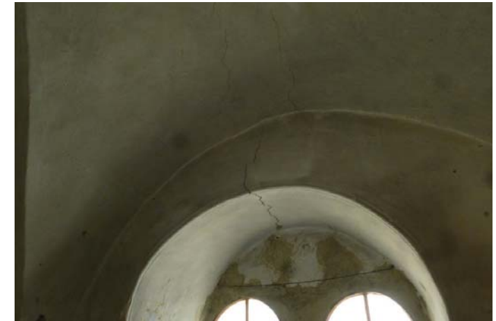
3. Observing any cracks and their progression over time can provide useful information on structural damages and suggest the need for emergency intervention.
