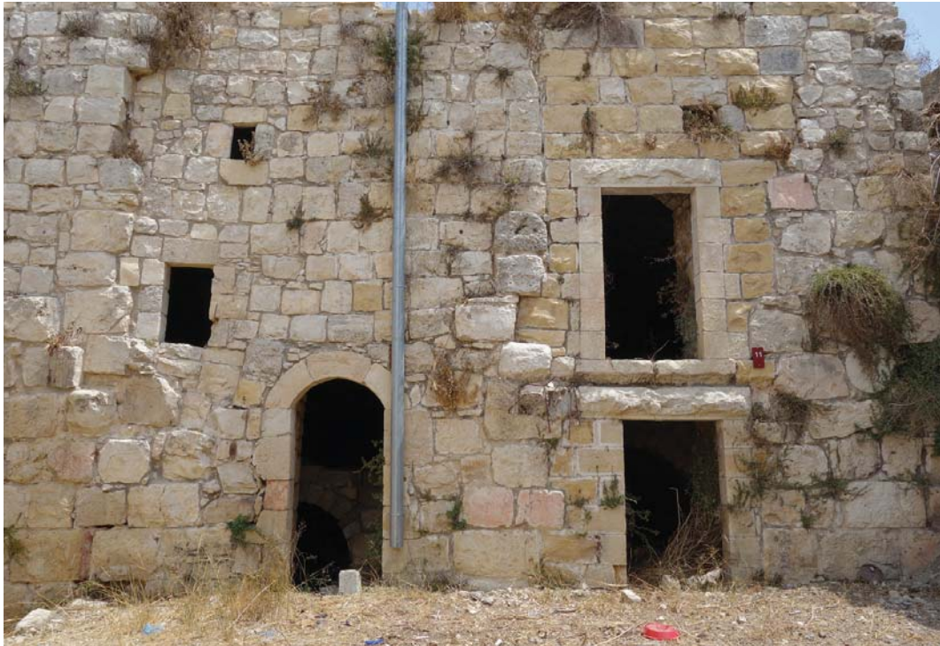
Visual analysis provides information on materials, the arrangement and height of stone courses, the thickness of the joints, possible cracks, etc.
