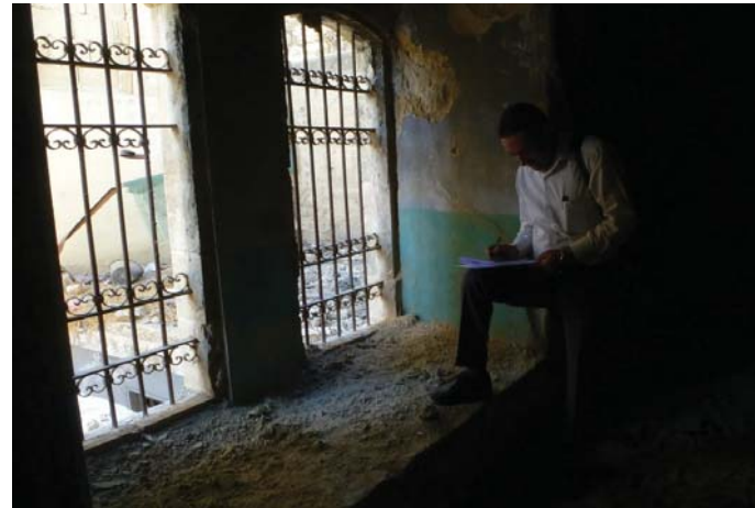
2. Periodic inspections of the buildings are key to identify possible risk factors and address them in order to prevent serious damages in the future.
