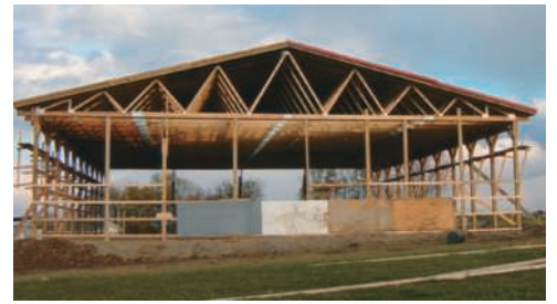
Photo 6.4 Because roof trusses, such as those shown, require support only at their ends, it is possible to construct buildings with large, unobstructed interiors.
