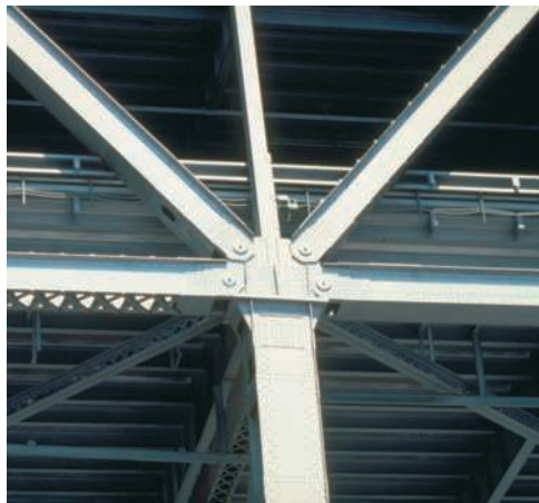
Photo 6.2 Shown is a pin-jointed connection on the approach span to the San Francisco–Oakland Bay Bridge.
