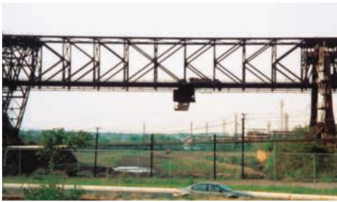
Photo 6.3 Two K trusses were used as the main components of the movable bridge shown, which moved above a large stockpile of ore. The bucket below the trusses picked up ore and redeposited it until the ore was thoroughly mixed. The ore was then sent to the mill for processing into steel.
